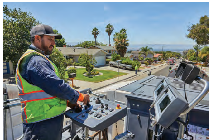
TOP: The Wirtgen cold recyclers can also be used as efficient, high-performance milling machines employing the up-cut process.
