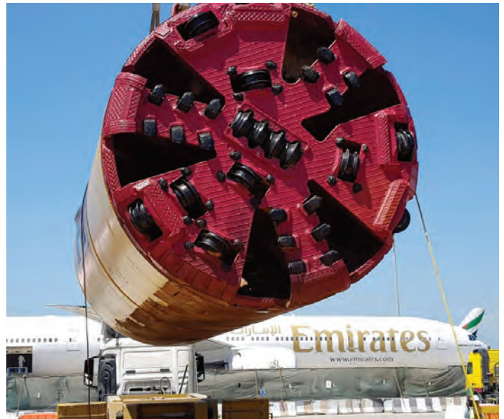
A Herrenknecht TBM, with a shield diameter of 3,025 mm, excavated three drives of a new 2,200-m-long stormwater drainage tunnel at the Dubai International Airport.
