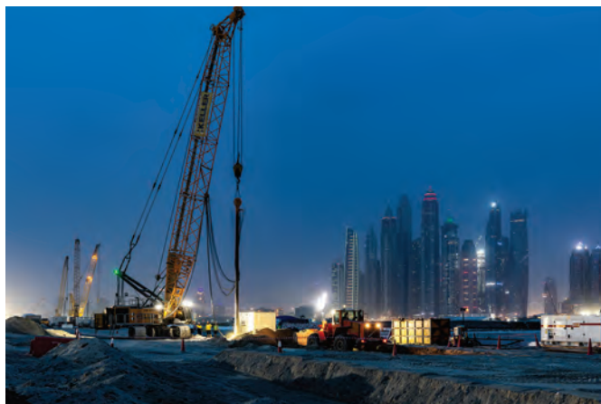
LEFT AND BELOW: A new harbour development featuring almost 2 mil sq m is currently underway in Dubai. For this project, Keller Grundbau GmbH is compacting more than 7 mil cu m of sand in an area of 380,000 sq m, with the help of a Liebherr HS 8130 duty cycle crawler crane.
